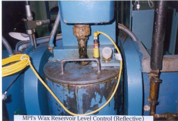
MPI's Wax Reservoir Level Control (Reflective) connected to a Jahnke press' refill port
